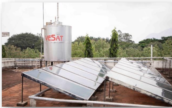
Solar Water Heater- Boys Hostel
