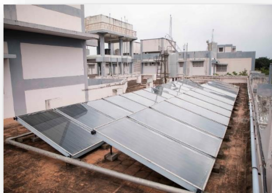
Solar Water Heater- Ladies Hostel 1
